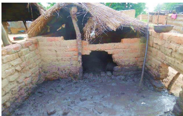
Figure 2 : Housing partially broken
